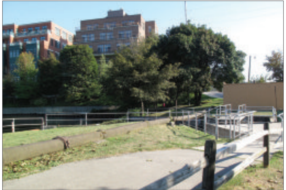
Crest of Union Street Dam: Fish ladder and utility building along with existing infrastructure functionality should be considered in any retrofit to the dam.
