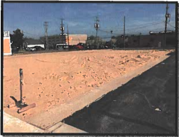
Figure 12. New Construction Sediment Deposit at the corner of W Front St and Pine St
