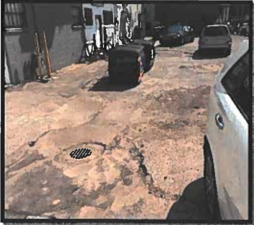
Figure 11. Sediment in Alley
