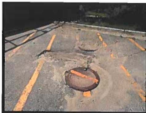
Figure 42. Sediment Deposit In Parking lot
