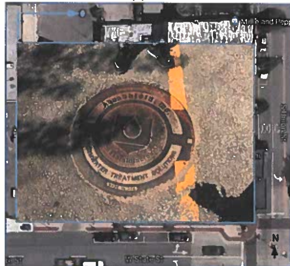
Hydrodynamic separator located in the parking lot of Panache Boutique.
