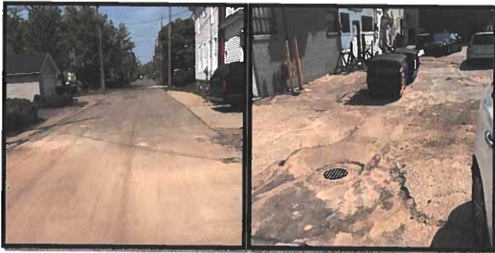
Figure 44. Sediment in Alley, Catch Basin
