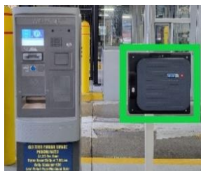
Figure 3: Shows the Old Town Parking Deck card reader and intercom location. Outlined in green.
