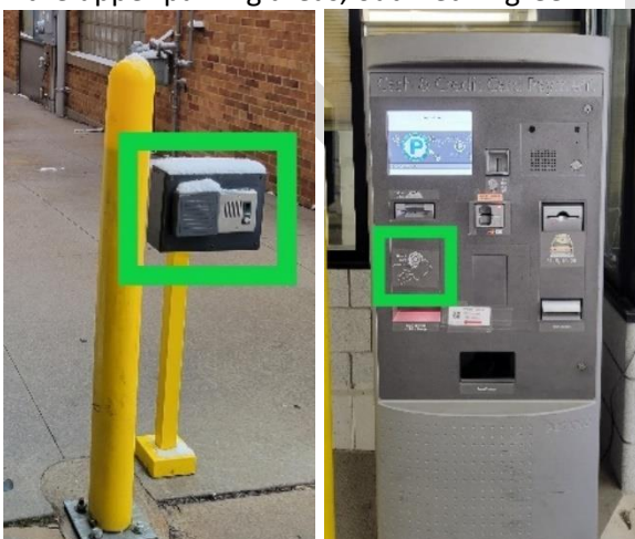
Figure 5 A, B: A(Left) shows the Front St. exit card reader and intercom. B(Right) shows the State St. exit card reader and intercom. Both outlined in green.
