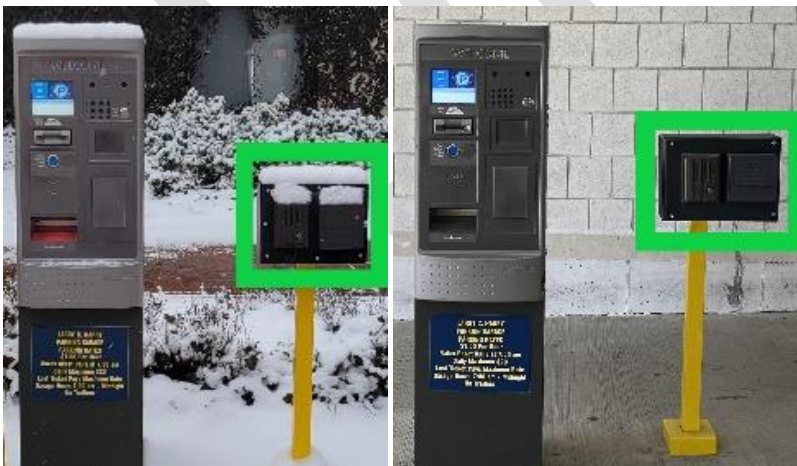
Figure 2 A, B: A(left) shows the front street entrance card reader and intercom, B(right) shows the state street entrance card reader and intercom. Both outlined in green.
