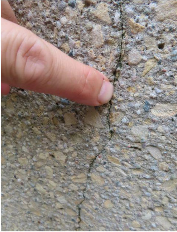
Precast Spandrel Panel Cracking — Close-up photo of the spandrel panel cracking.
