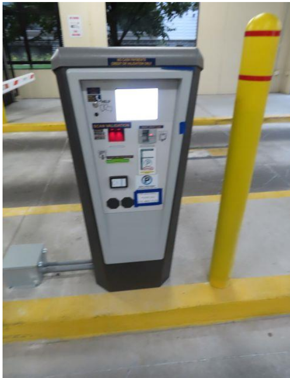
Closeup of Revenue Control Equipment — Revenue control equipment at exit from structure.
