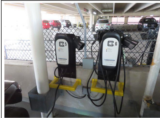
Typical Electric Vehicle Charging Station — EV charging stations are typically found at the south end on the east bay on the supported levels.
