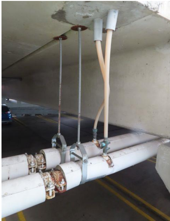
Level 4 Center Bay Glycol Heating System — Piping and connection of glycol heating system at underside of Level 4 in the center bay.
