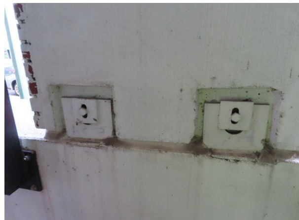
Precast Spandrel Panel Steel Connection Plates — The exposed steel plates have been painted and appear to be in good condition.
