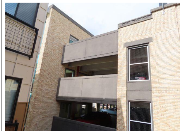
South Façade at Stair Tower — South façade at southwest stair / elevator tower. Photo shows precast spandrel beams with no in-laid brick.
