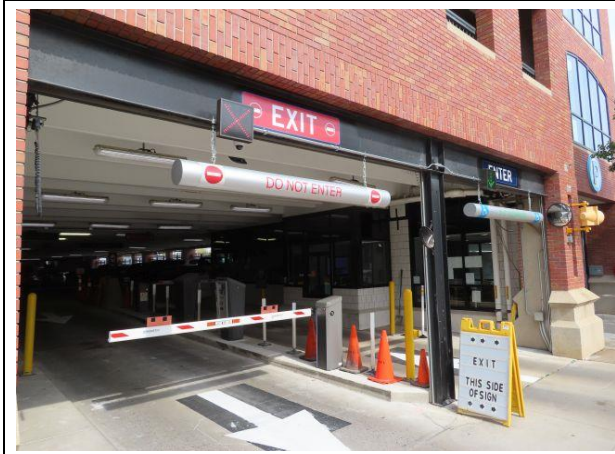
South Entry / Exit PARC Equipment — This photo shows the parking access and revenue control (PARC) equipment at the south entry / exit.
