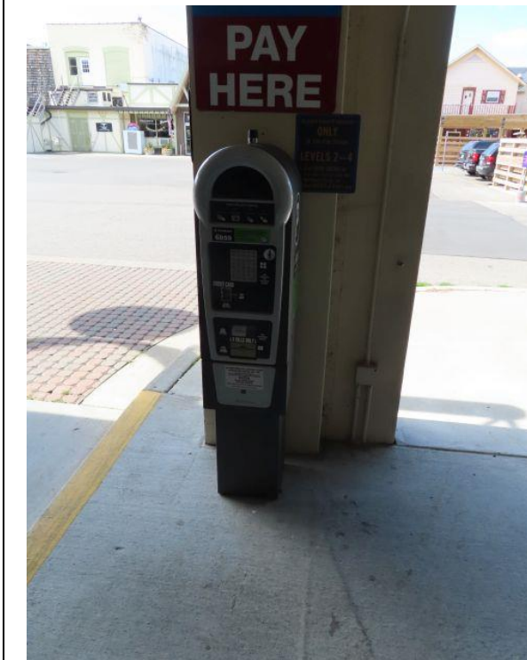
Revenue Control Equipment — Pay on foot station at northwest corner of structure on Level 1.
