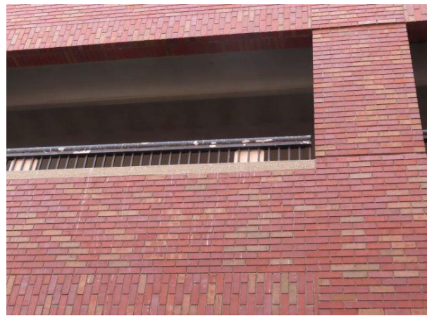
Perimeter Railings Peeling Paint — The railings / fences around the perimeter of all levels are painted metal. Several areas of peeling / missing paint were observed. We recommend cleaning / painting these railings.
