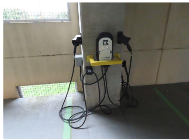
Electric Vehicle Charger — Electric vehicle charging stations are typically found at the north end of the structure on each supported level.
