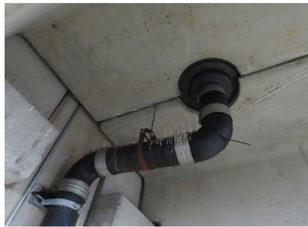
Floor Drain & Piping — Typical supported level floor drain with cast-iron piping. This piping may require future replacement maintenance as it corrodes.
