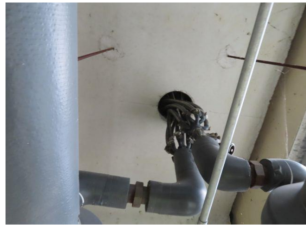
Glycol Heating System at Level 4 East Bay — Underside of Level 4 east bay showing the glycol heating system for the east bay. This system is only on the Level 4 east bay and is used to melt snow and ice on the sloped bay.
