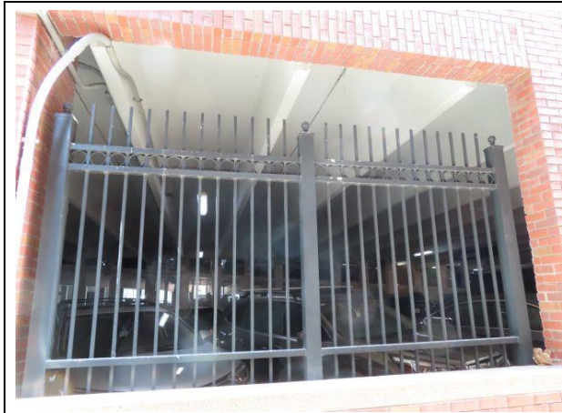
Level 1 Fencing – Ornamental metal fencing is provided in the openings at Level 1.
