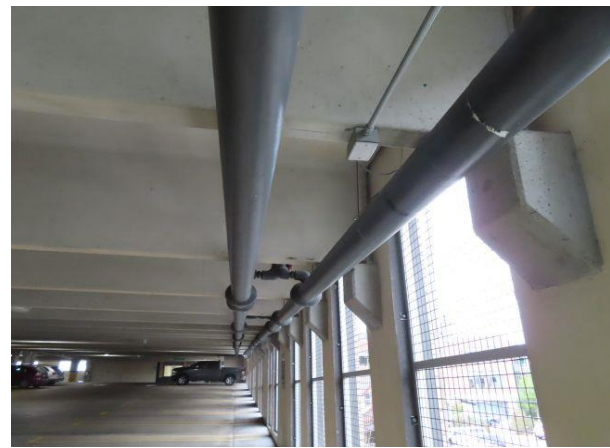
Piping for Level 4 Heating System — Underside of Level 4 east bay showing the piping for the glycol heating system.
