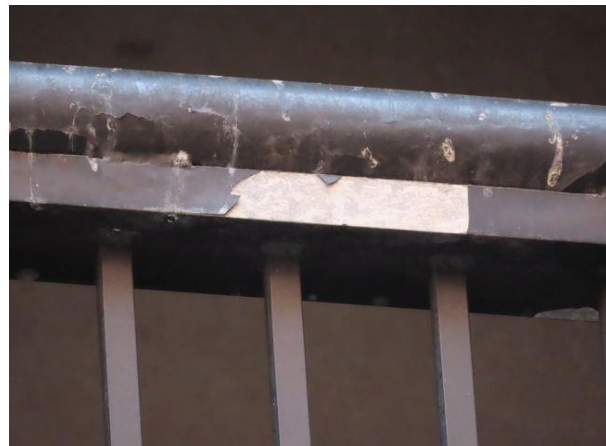
Perimeter Railings Peeling Paint — Close-up photo of the peeling paint.
