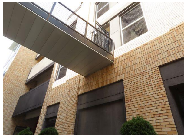
Underside of Bridge at South Facade — Underside of bridge from Level 2 of parking structure to housing located south of the structure.
