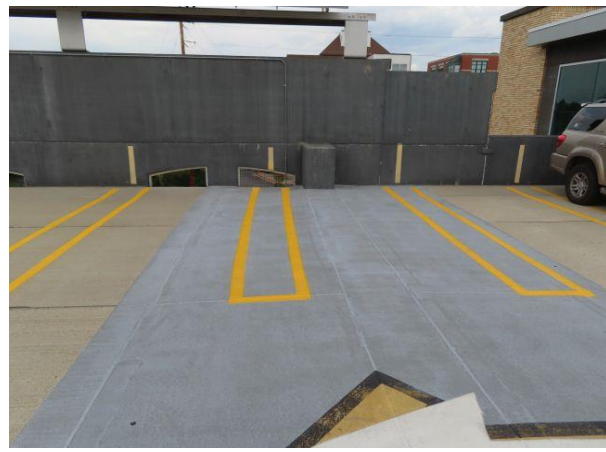
Crossover Traffic Bearing Membrane — Traffic bearing membrane installed over one of the crossovers on Level 4. All supported levels of the structure have traffic bearing membranes installed over the cast-in-place washes at these crossovers.
