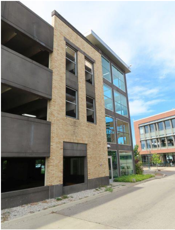
Northeast Stair Tower — Northeast corner of the structure showing façade and the stair / elevator tower.
