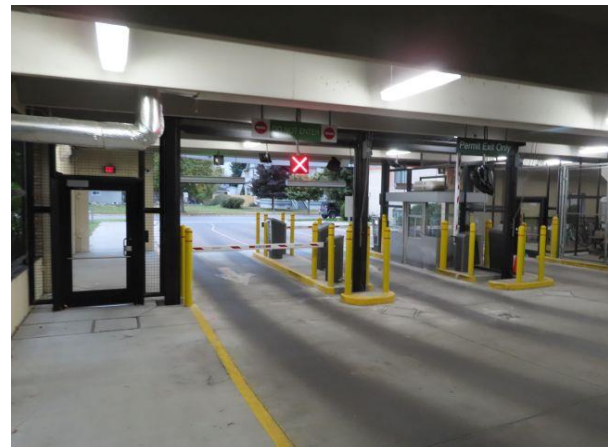
South Entry / Exit PARC Equipment — South entry / exit point to the structure showing parking access and revenue control (PARC) equipment.
